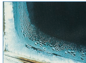
Window condensation can fuel mold growth.
